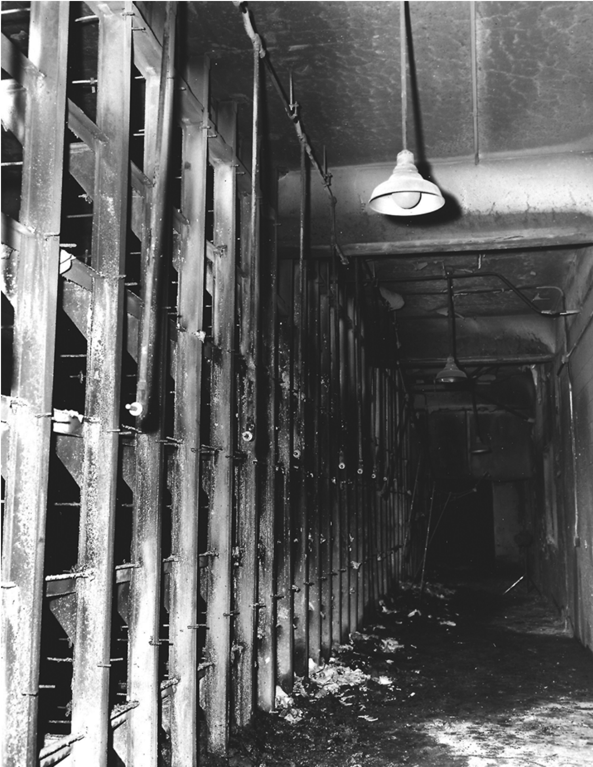
Chapter 7. Room 180 in Building 771 at the Rocky Flats atomic bomb plant in Colorado. This is where the fire started on September 11, 1957, in the glove box, middle left in the picture. Gloves have been turned inside out and are hanging down.
